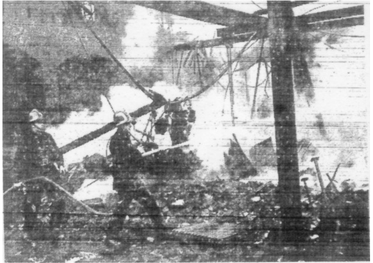
THIS was the scene today at the works block of Mellows and Co. Ltd., Corporation Street, Sheffield: Firemen play water on the smouldering remains of the gutted building.
